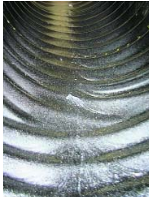
FIGURE 6. Polymerized asphalt over galvanizing after test run 3.
