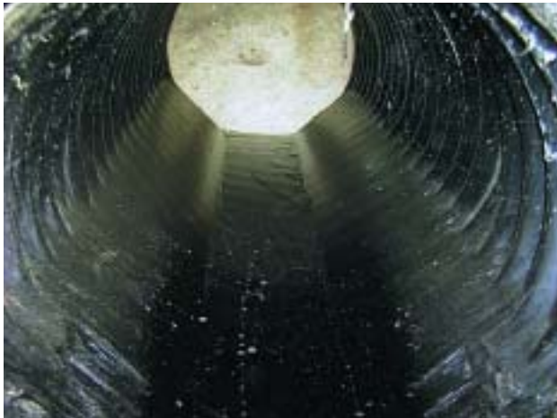
FIGURE 5. Asphalt paved pipe after test.
