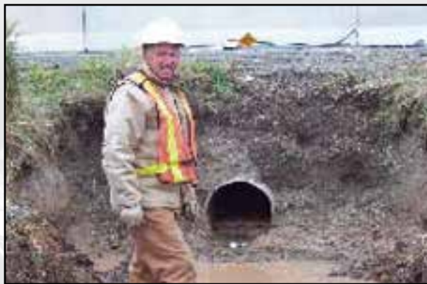
CULVERT SILTED WITH DE-ICING SALT & SAND
