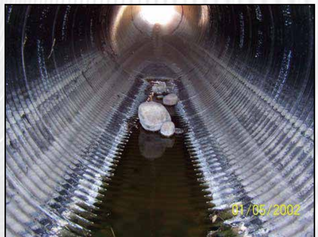
AS WINTER RUNOFF EVAPORATES, ROAD SALT IS CONCENTRATED AND DEPOSITED ON PIPE SURFACES. ALTHOUGH VISIBLE ON THE BLACK POLYMER LAMINATED SURFACE IT HAS NO EFFECT ON THE LAMINATE OR THE UNDERLYING GALVANIZED STEEL.
