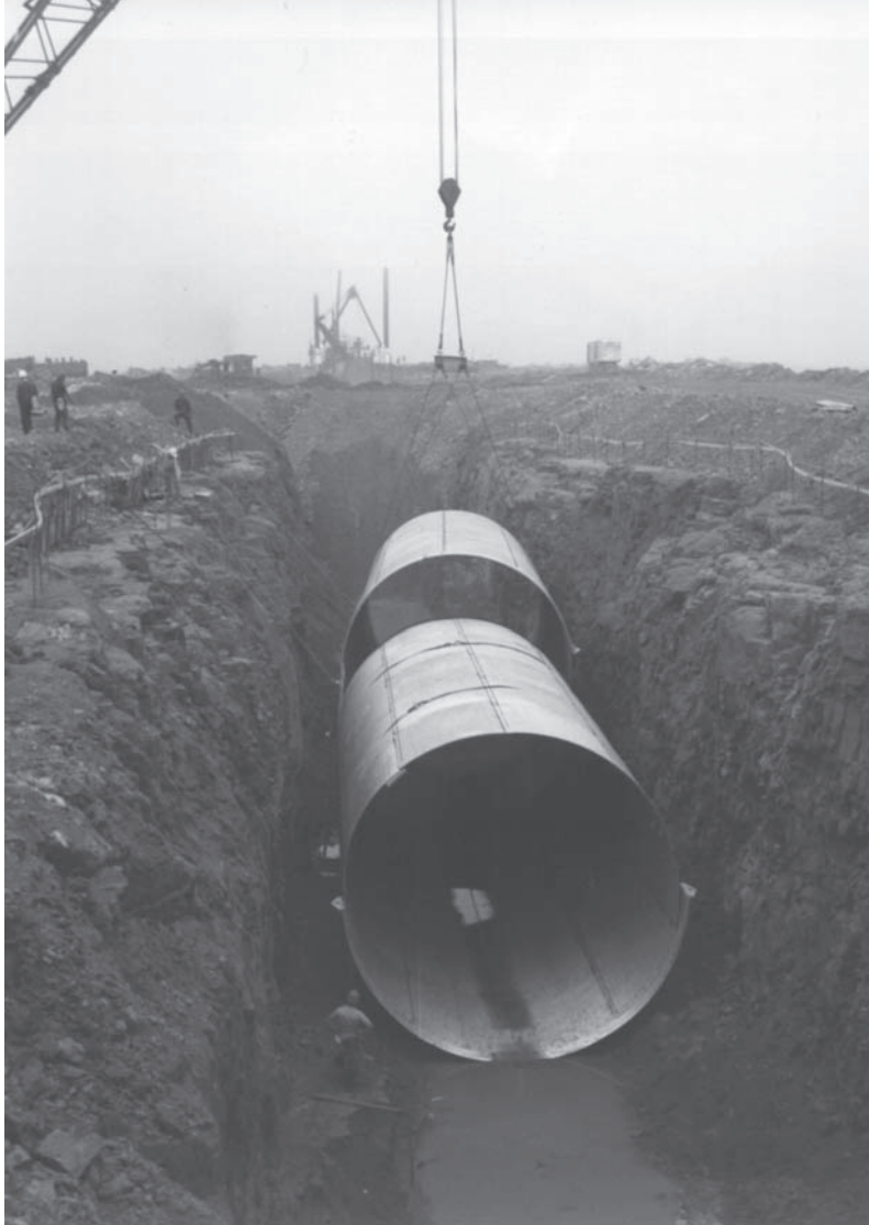
Versatility of steel in sewer construction is typified by application of large diameter structural plate pipe.
