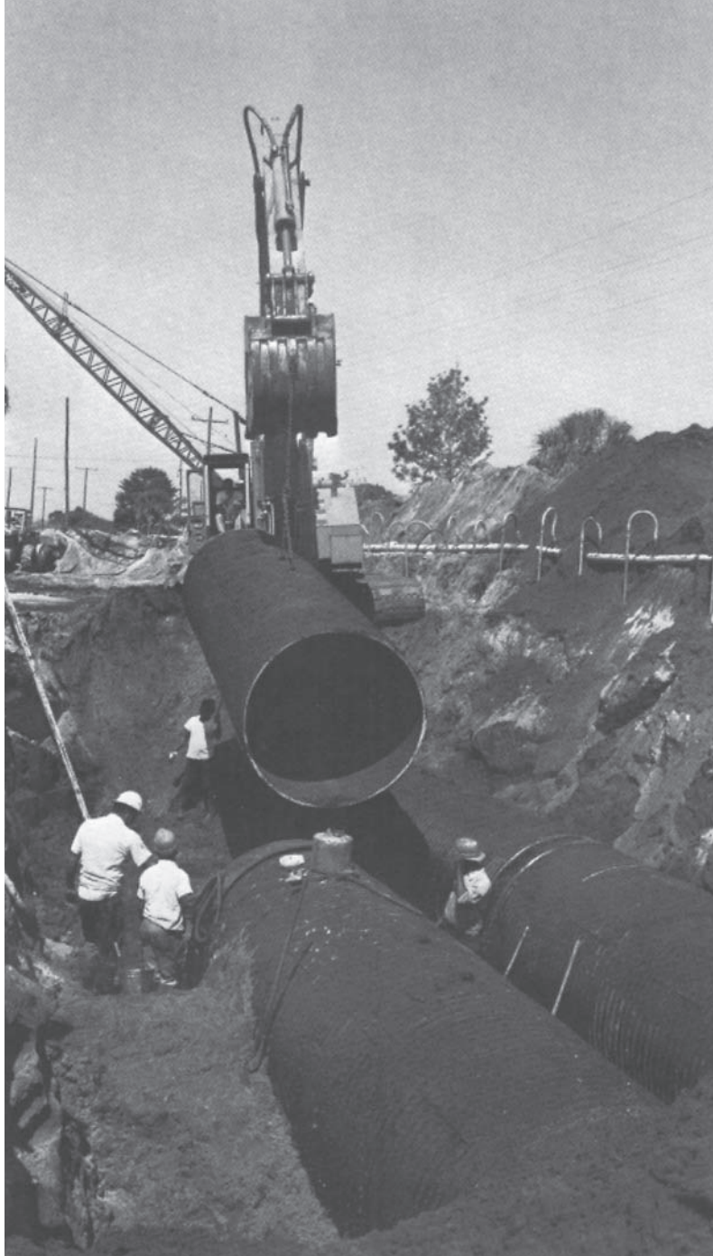
Well points and wide trenches were necessary to install full bituminous coated and full paved CSP in this unstable ground.
