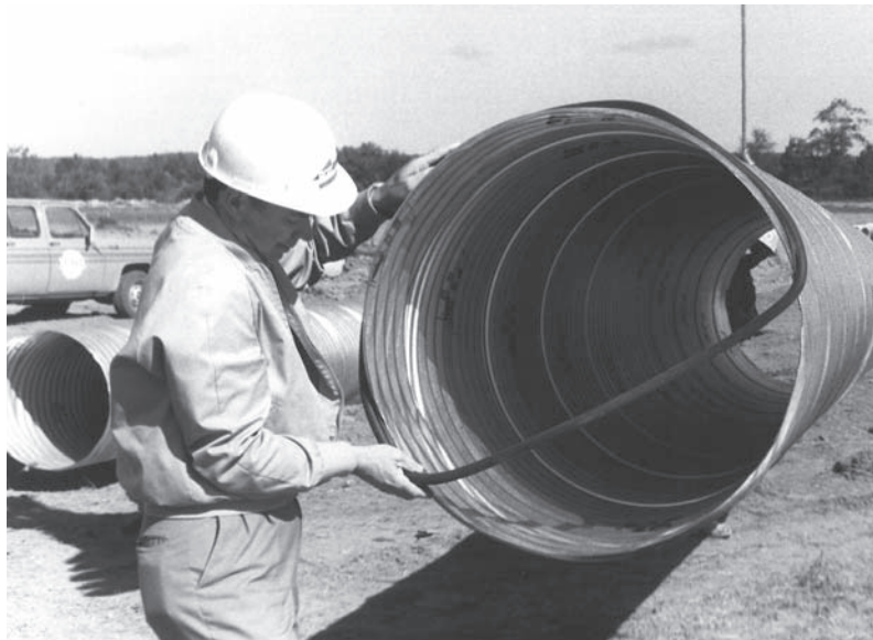
"O-Ring" being placed over the end of the pipe and recessed into the end corrugation.
