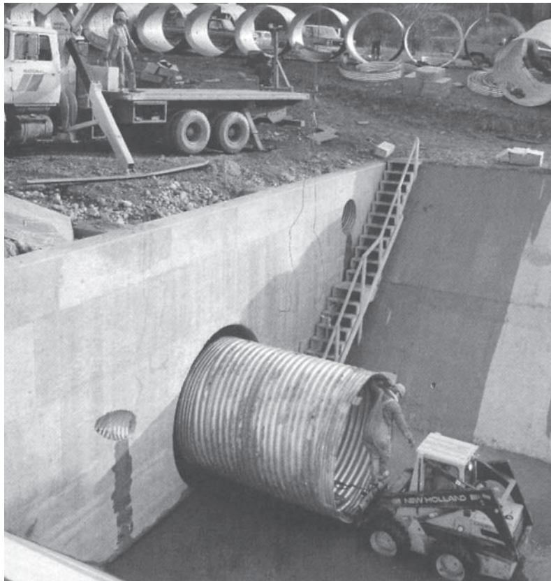
A rehabilitation technique called "Sliplining". A 2400mm dia. CSP being sliplined into a 2800mm dia. failed concrete pipe.
