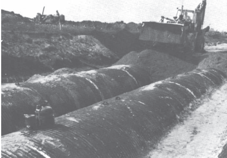
Philadelphia Airport expansion again calls for CSP storm sewers. Corrugated steel pipe was installed 25 years before in an earlier expansion.
