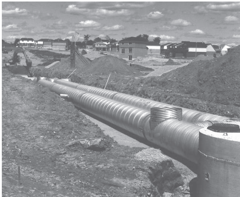
A twin run of 1200 mm diameter CSP provide an underground stormwater detention system for a site in Southern Ontario.
