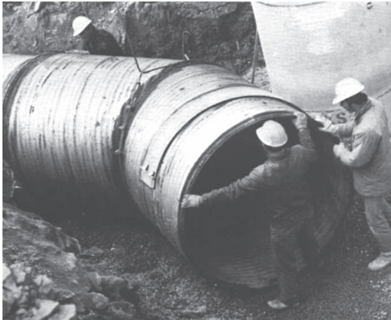
Pre-fabricated miter section of CSP is lowered into place to match bend in trench.
