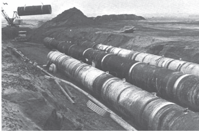
3000 mm diameter, 76 x 25mm full bituminous coated and full paved 1500m installed as stream enclosure for runway extension.
