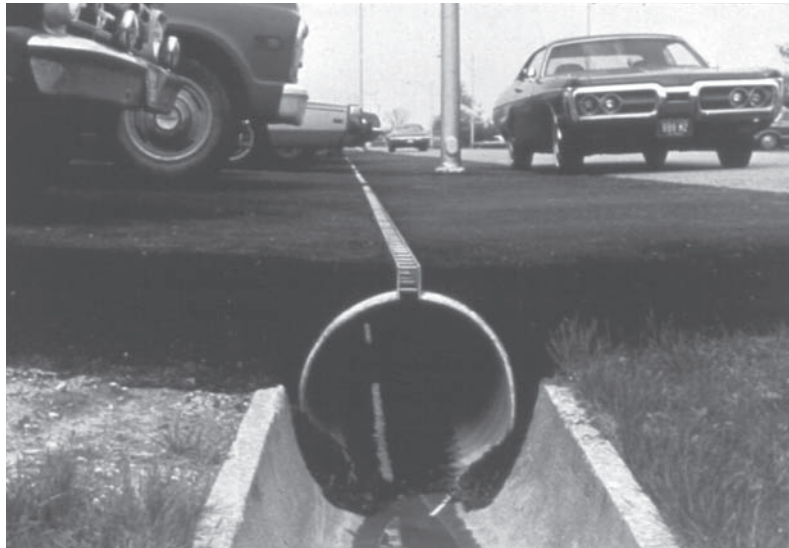
Slotted drain carries water away from parking area.
