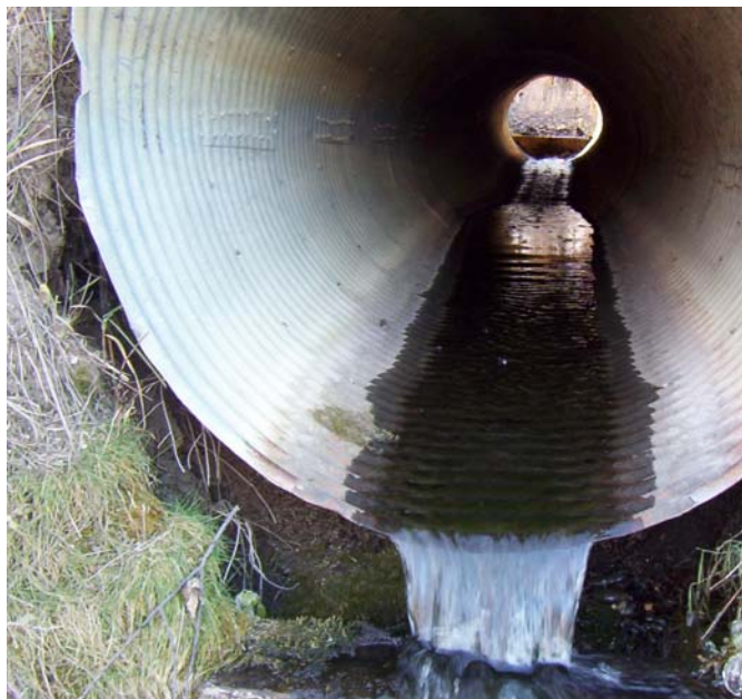
Protective Scale on Older Culvert
