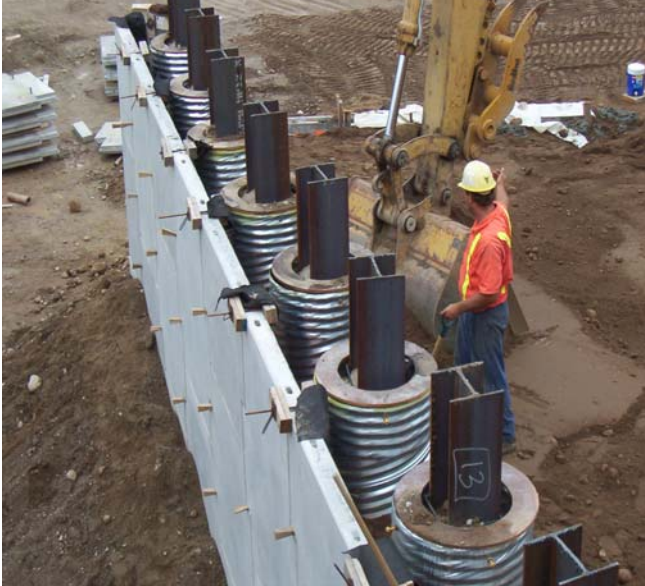
Minimal Clearance to Retaining Walls
